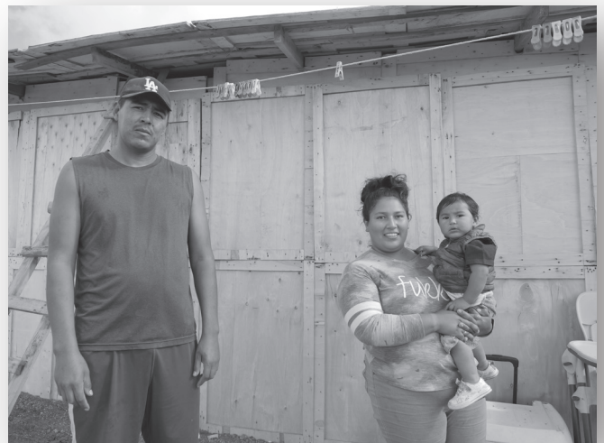
Part of the roof of their home blew off during a recent storm
