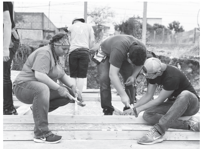
Building a home for a family in need can also build relationships on the team
